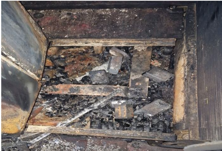
Fig. 4.12. Image of the burst capacitors.
