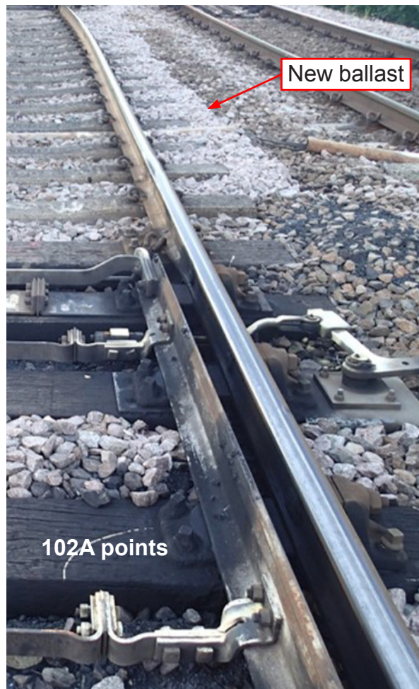
Figure 13: Area of ballast dressing in the six-foot between 102A and 101B points
