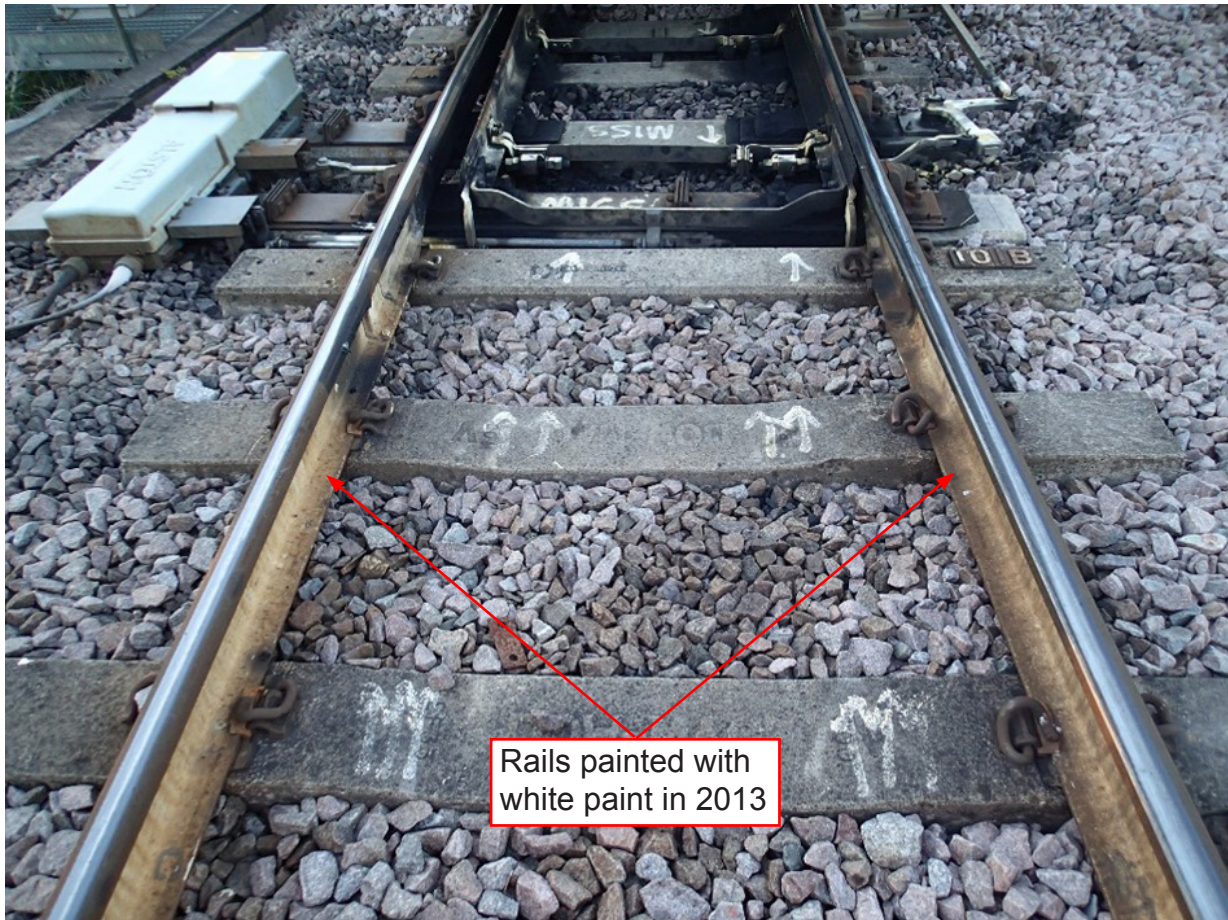
Figure 11: Sleeper tops above ballast at toe of 101B points
