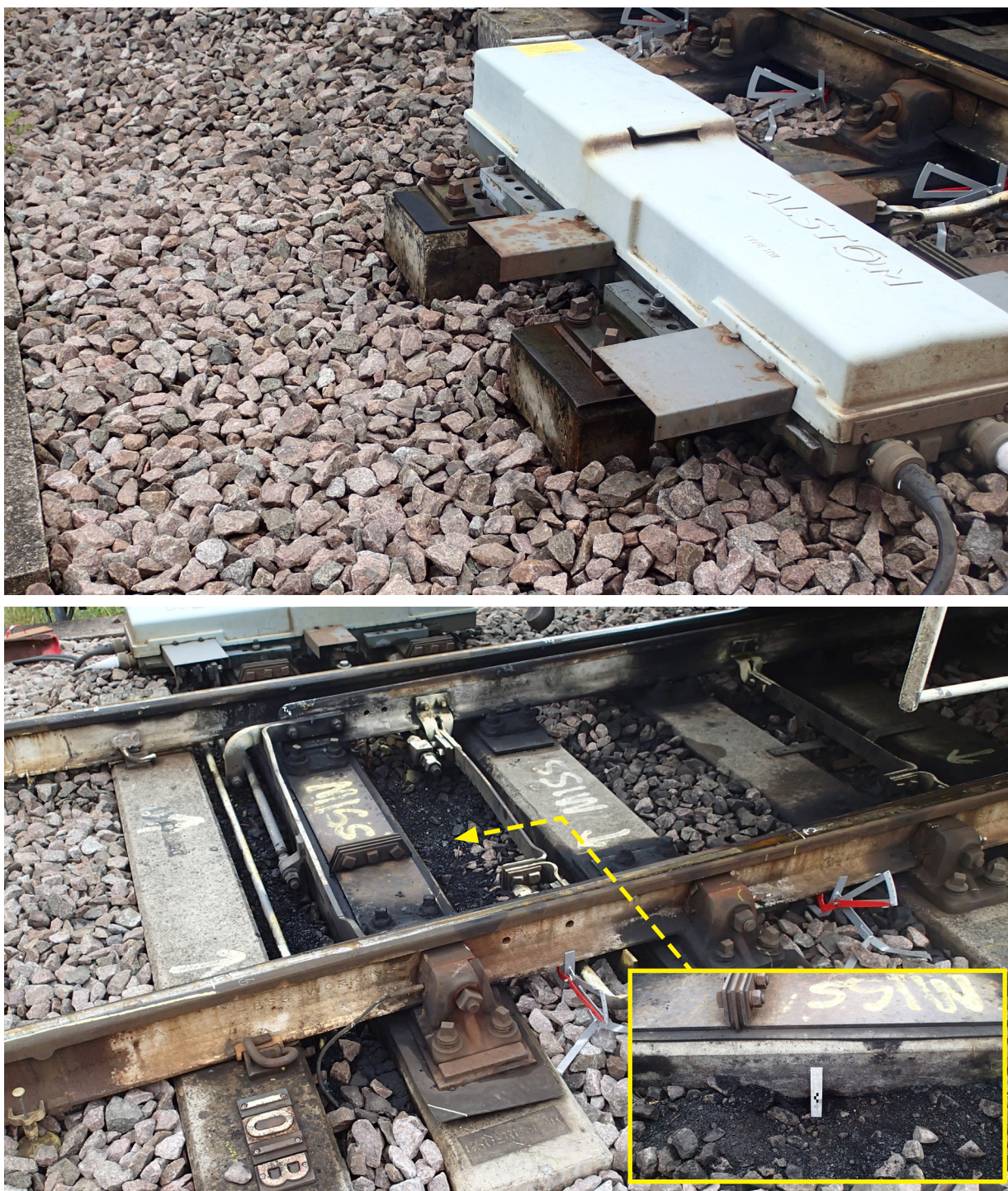
Figure 9: Ballast support at the ends of 101B point motor bearers and in the 'cribs' at the toe of the points
