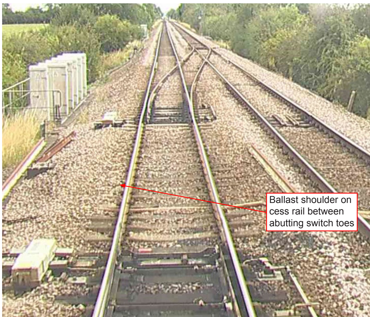
Figure 12: Ballast shoulder in plain line section between 102A and 101B points, captured by the forward facing CCTV camera on Network Rail's track recording train, August 2014 (image courtesy of Network Rail)
