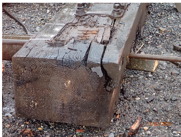
Figure 20: Timber 1L before cutting, but following removal of the first baseplate beyond the point of derailment
