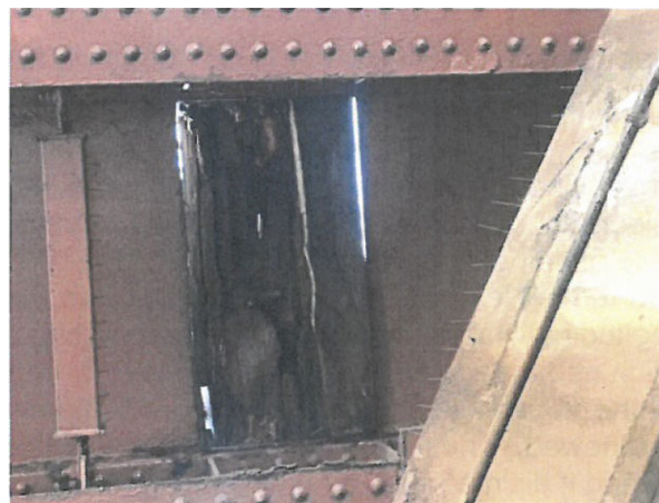
Figure 4: damaged timber from below. Daylight is visible.
