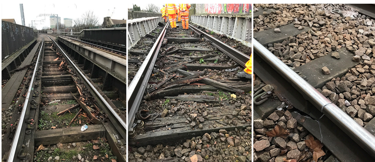
Figures 9, 10 and 11: Examples of track damage between point of derailment and location where train stopped
