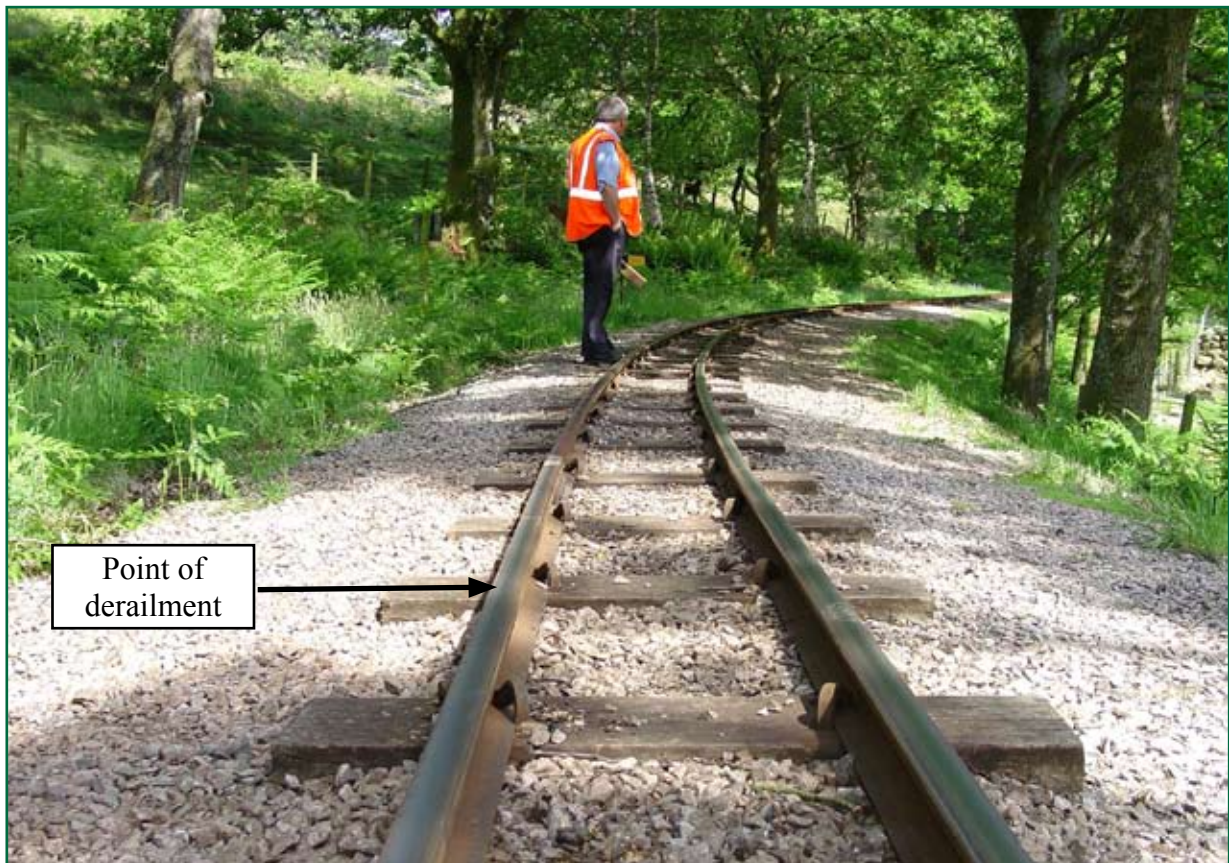
Figure 2: Site of derailment at Spout House Curve.
