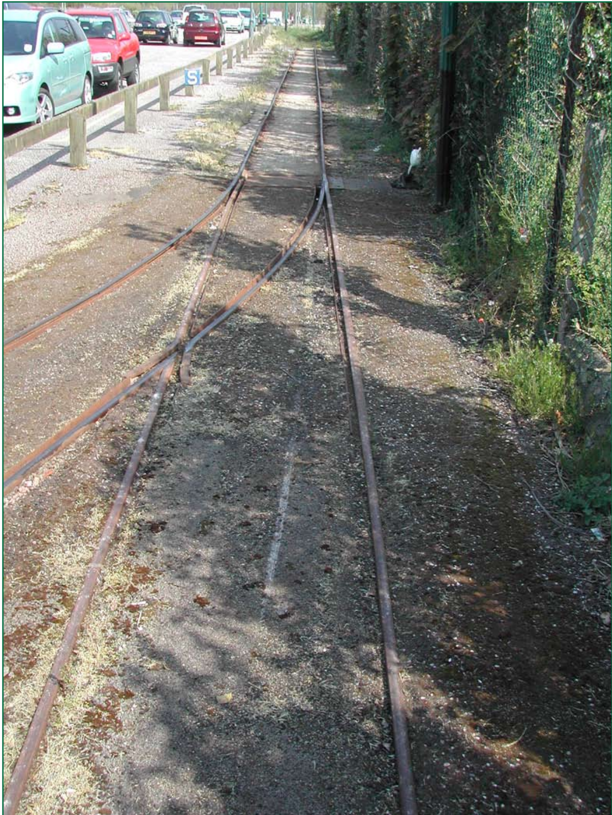
Figure 6: Marks from derailment
