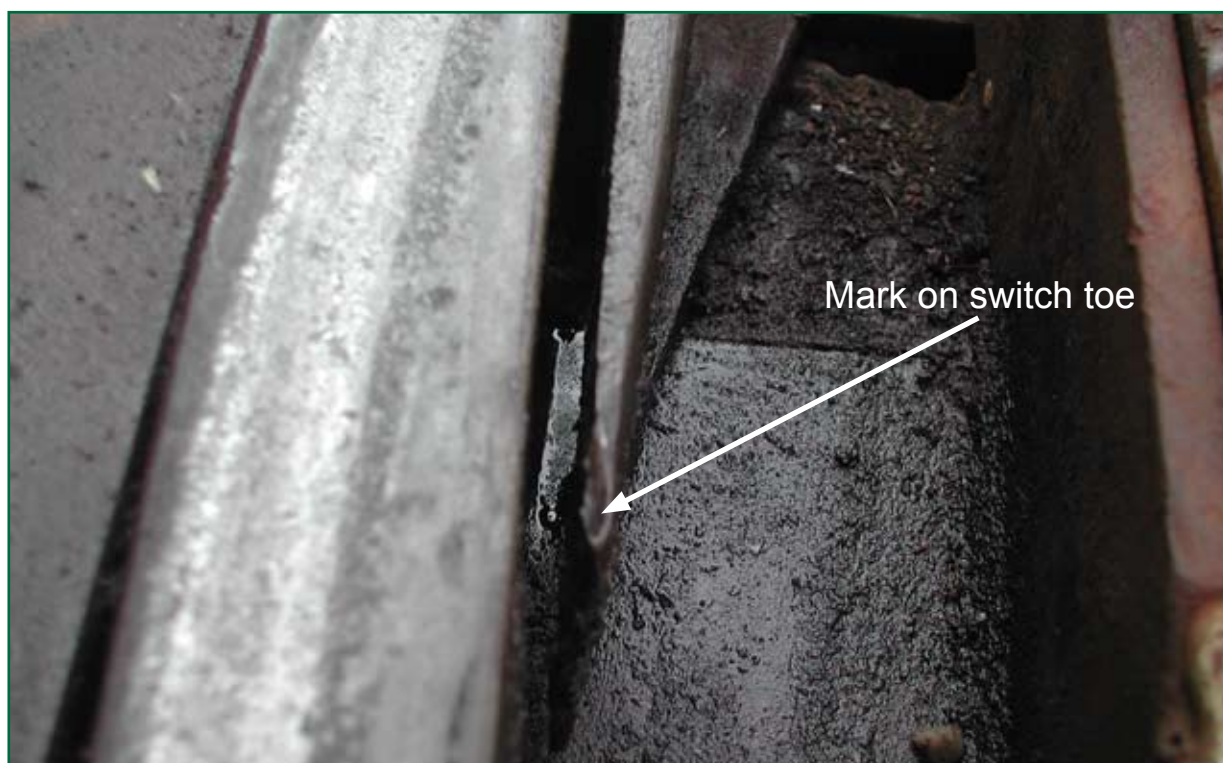
Figure 7: Mark on switch toe
