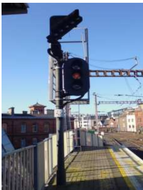
Figure 99 – Signal CY91 (Platform 5)
