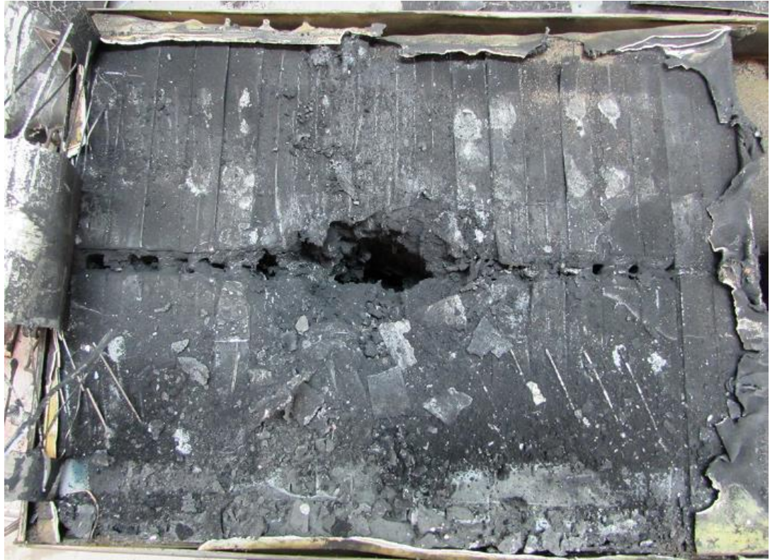
Figure 3: The state of the C2 capacitor
