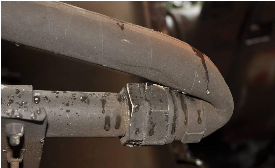
Figure 17 Detail of the kinked air hose (source: Bregenz CID)
