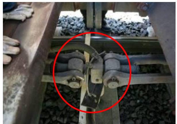
Figure 46 Securing cable with plastic sleeving
