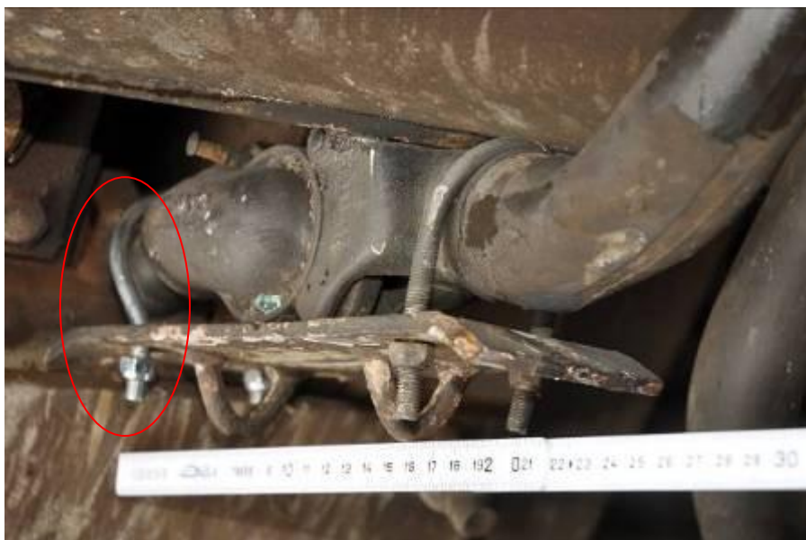
Figure 39 Metal plate with a new U-bolt
