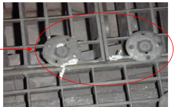
Figure 11 Detail of the signs of shear
