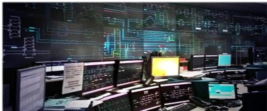
Traffic control room
