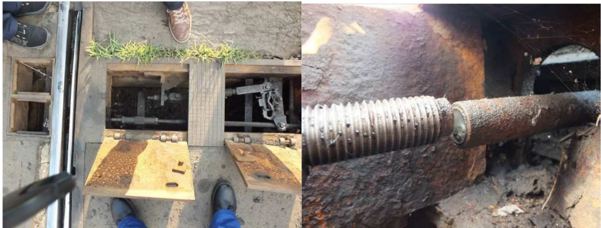
Figure: Fracture of the short pull rod
