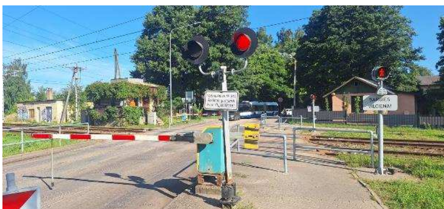
Figure 15. Pedestrian movement control barrier installed after the accident. View from the Rostokas iela side
