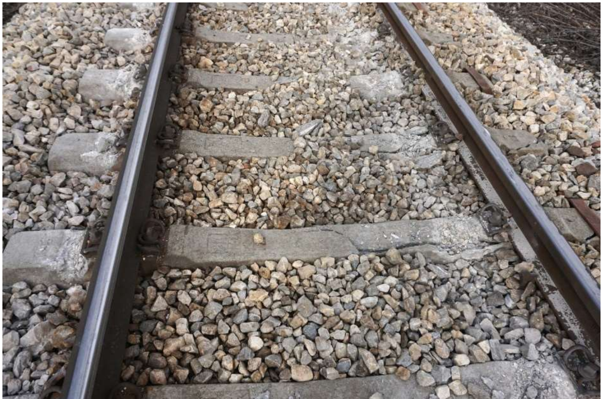
Figure 4.2.9.1: Damaged and broken sleepers
