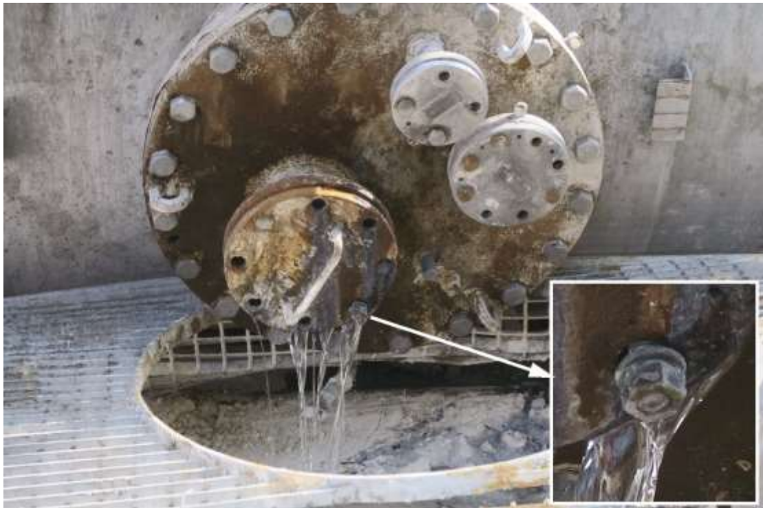
Figure 4.2.11.1: Acid leakage at the filling lid
