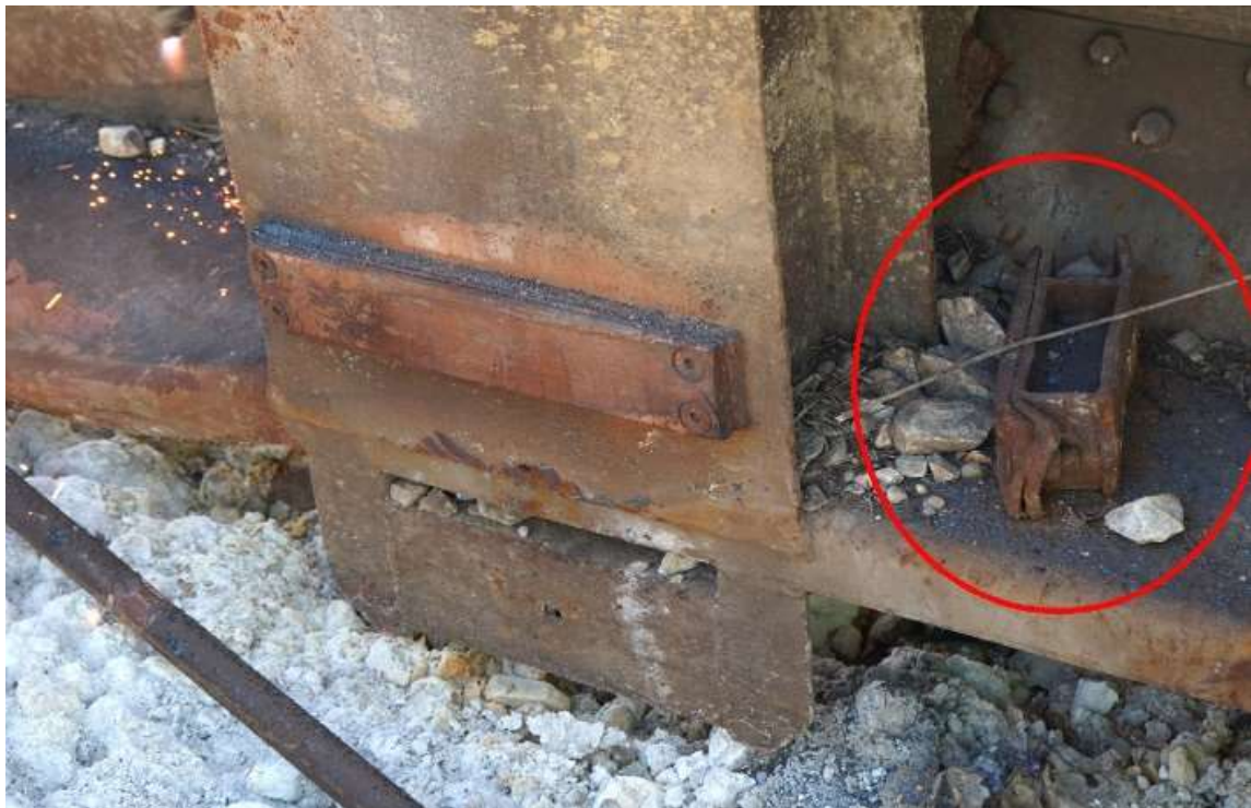
Figure 4.2.13.6: Position of the torn lower slide bearers
