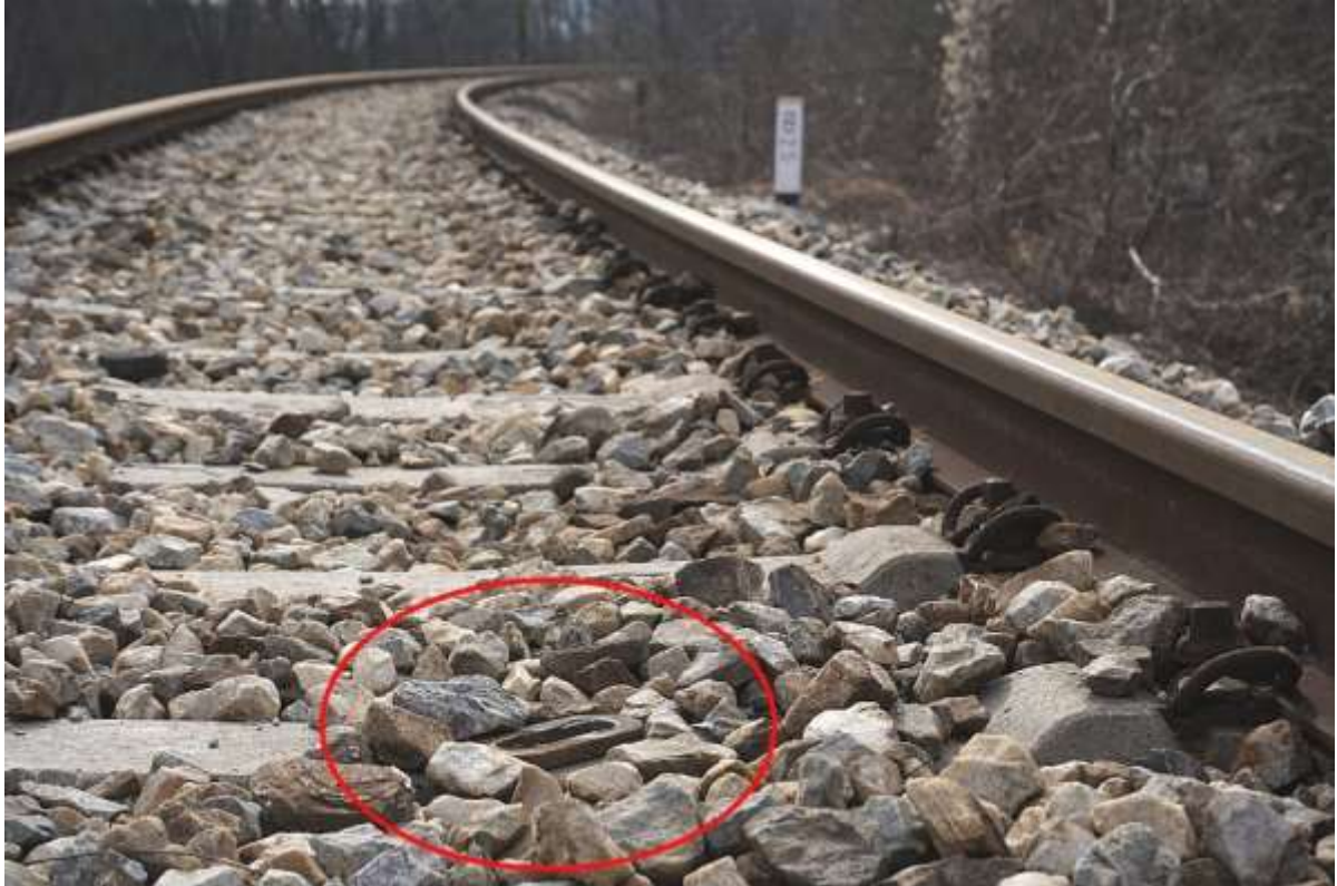
Figure 4.2.9.3: Fallen out suspension link
