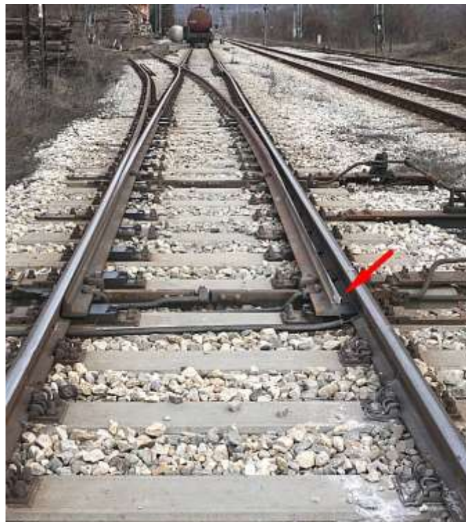
Figure 4.2.10.2: Broken switch blade and wheel marks on the switch point of switch No. 4 at Vrčin station
